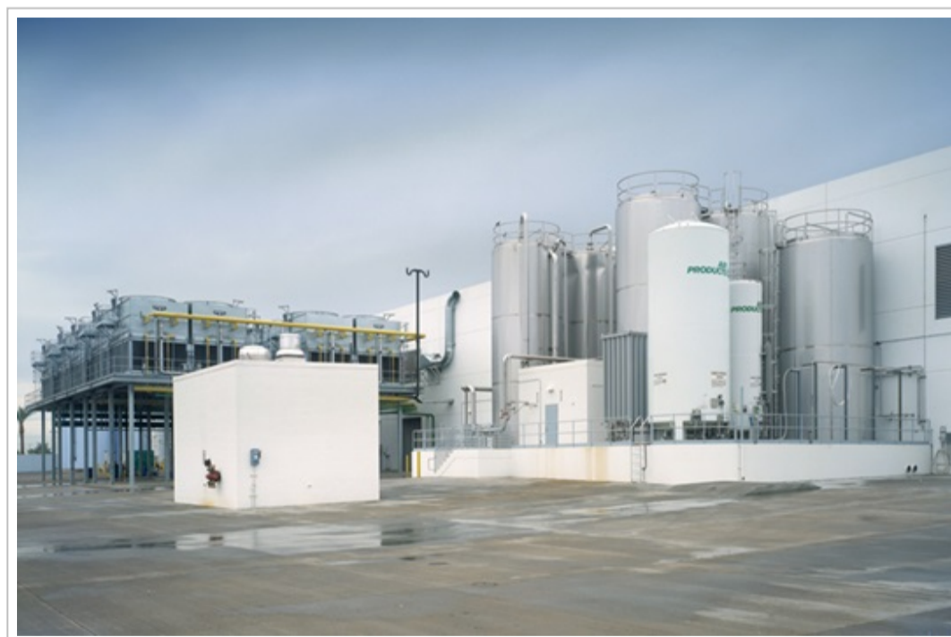
At refrigerated facilities, a significant amount of site area is required for refrigeration equipment and storage silos that supply the manufacturing process. Ware Malcomb
