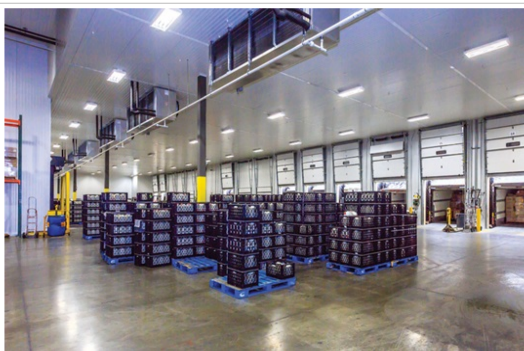
A cold dock with pallets waiting to be loaded into refrigerated trucks. Ware Malcomb
